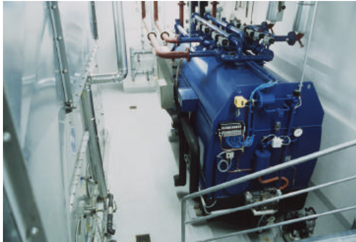
Figure 2.4. Adsorption chiller from the manufacturer Nishyodo; the machine is used for solar-assisted air-conditioning of a laboratory building at a hospital in Freiburg/Germany
