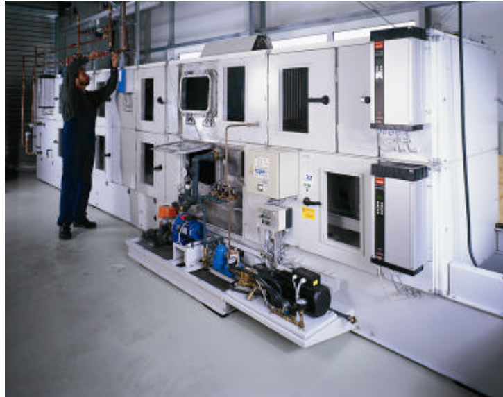
Figure 3.3. Example of a desiccant air-handling unit with desiccant wheel (nominal air-flow of 4500 m 3 /h).
