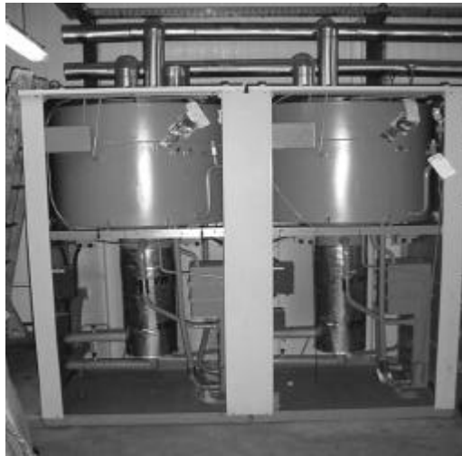
Figure 2.2. Photograph of a 52 kW single-effect absorption chiller installed in a plant for solar air-conditioning of a wine cellar in Banyuls/France.
